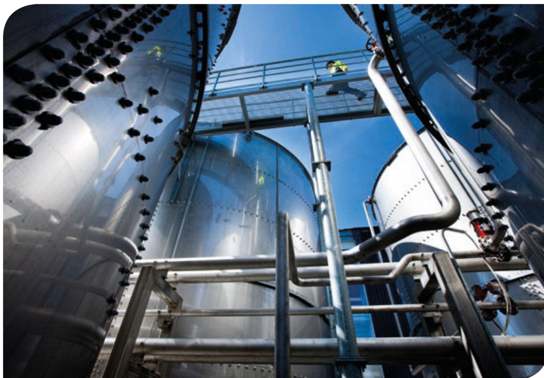
Our Greenmills AD facility in the Netherlands
