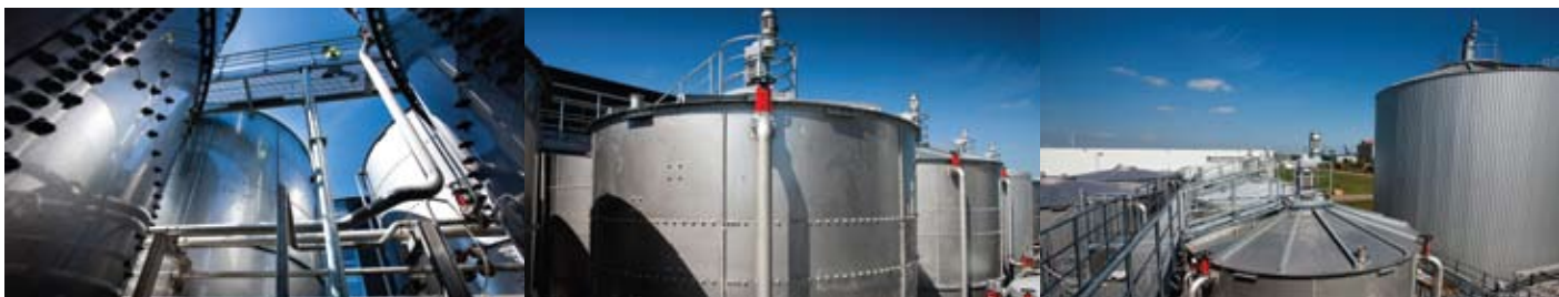
The Greenmills wet Anaerobic Digestion (AD) facility in Amsterdam will be the largest in Europe
